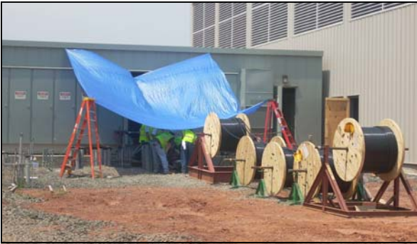
Switchgear meets cable
