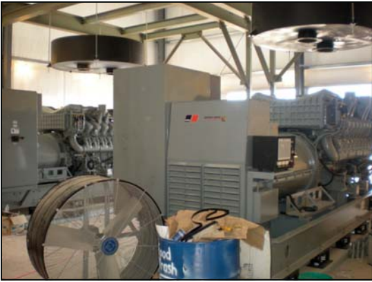
HVAC Gensets installed with mufflers and SCR support steel
